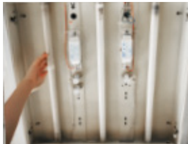
2. Disconnect wires and remove the original fluorescent tube(s) and ballast from the existing fixture. (Recycle tubes according to state specific recycling guidelines).
